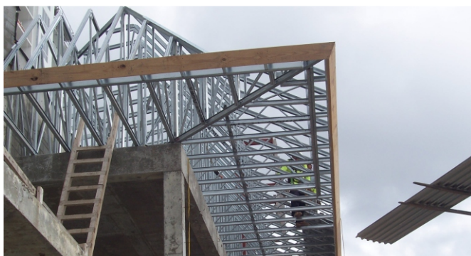
The facility incorporates many trusses to help create its distinctive appearance. “We had to be very creative with our designs,” says Scott Stanley, president of truss fabricator Scosta Corp.
